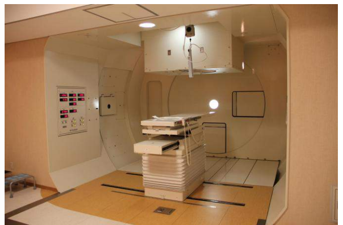
Proton Beam Treatment Room
